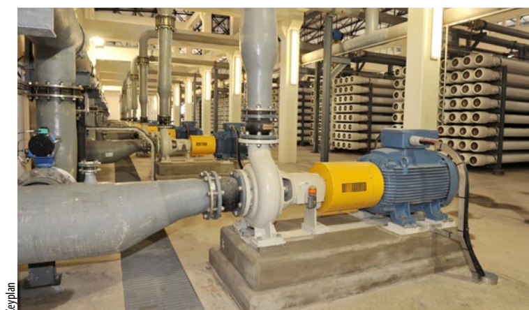
Top left: The low-pressure feed pump gallery for the seawater reverse osmosis plant.
