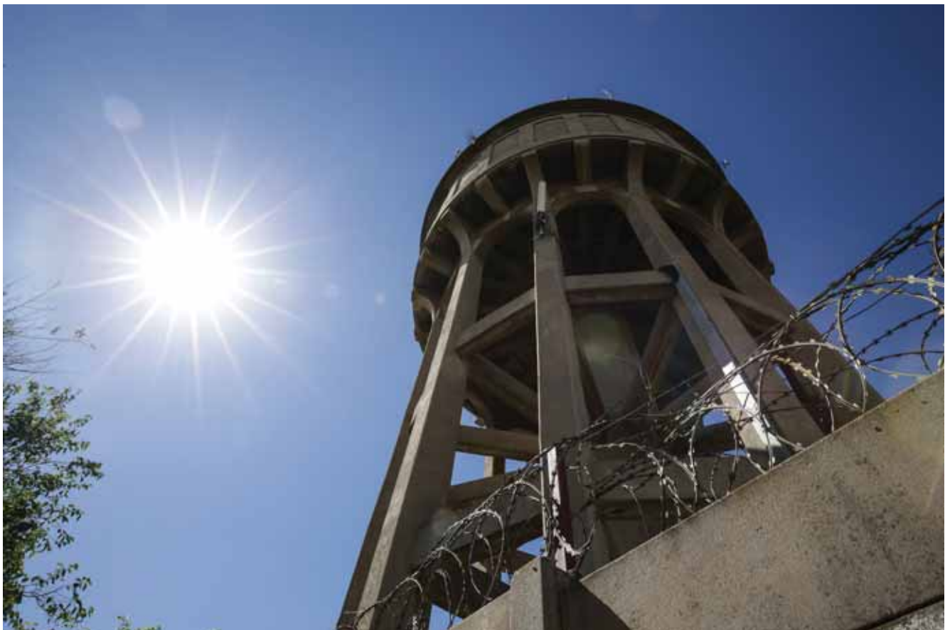
Johannesburg's connection with water goes much further than its water reservoirs.
